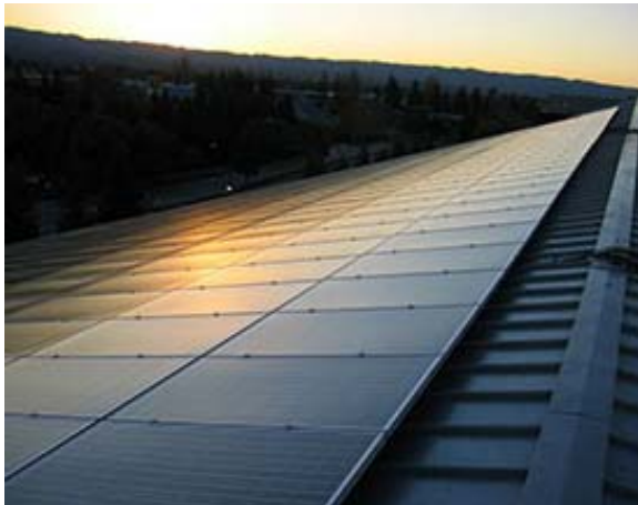
Estee Lauder Aramis Facility, Oakland, NJ. 600 KW solar photovoltaic array
