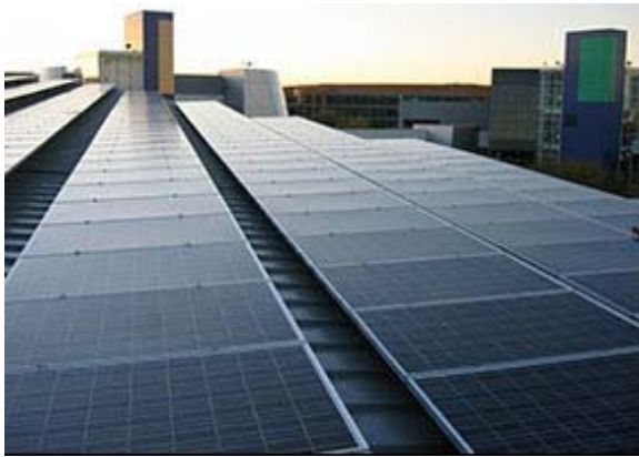
Google Campus, Mountain View, CA. 1.6 megawatt Photovoltaic array
