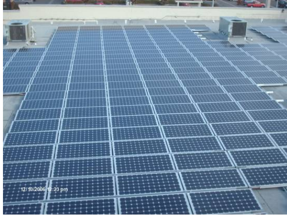
Typical 63 kW system on a Walgreens Drug Store
