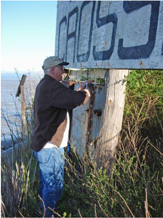
Tom opens 480 volt electrical panel
