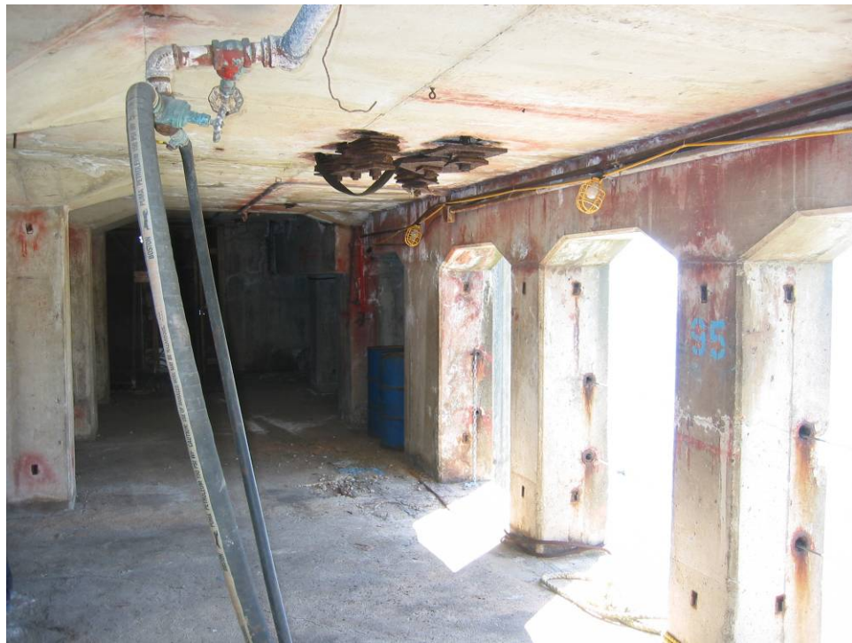
The gallery at Shipyard 3 under the area to which the whirly crane will be relocated and in which a new foundation will be constructed to support the relocated rail
